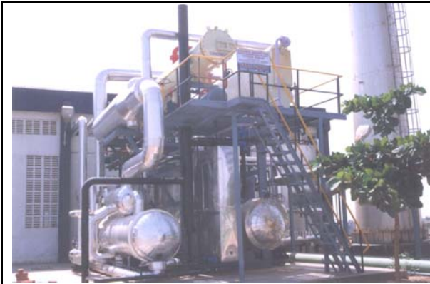
Figure 5 -Typical View of Ammonia Absorption Refrigeration Plant - "System Borsig" [1]
